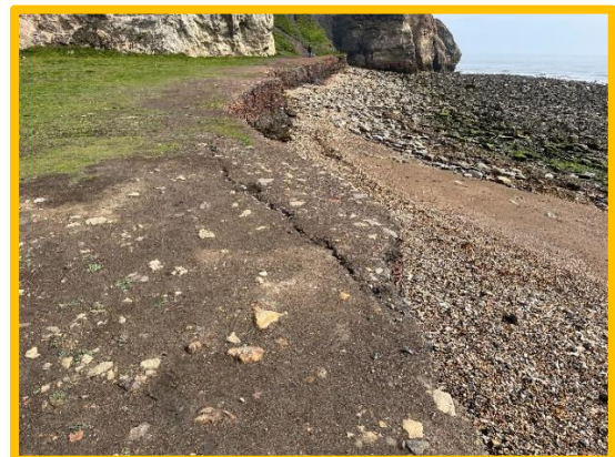
Tension cracks in actively eroding colliery spoil (/0103C07)
