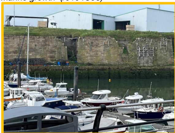
Gaps between blocks at Seaham North Dock (/0104C12)
