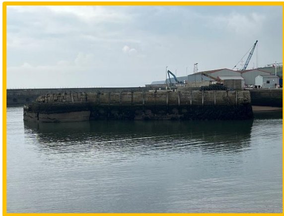
Loss of blocks and open joints (/0104C09)
