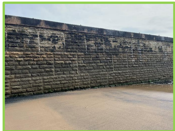
Seaham Harbour North Pier Inner Face (/0104C03)
