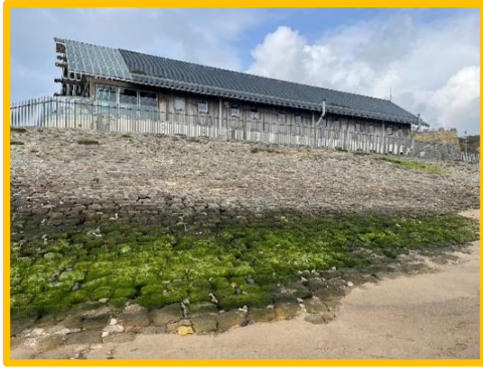
Open joints and vegetation growth on masonry revetment. High sediment levels (/0104C05)
