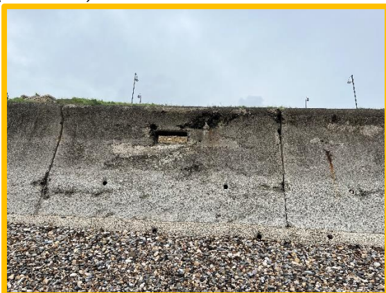
Heavily damaged section of sea wall to the south (/0102C01)
