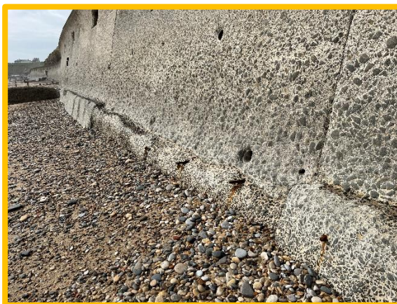
Heavily abraded wall exposing reinforcement (/0102C01)
