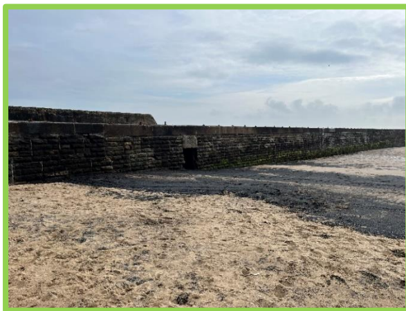
Seaham Harbour North Pier Inner Face (/0104C03)
