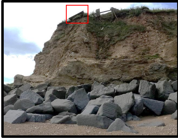
Erosion affecting fence line of properties to south Dawdon Dene Outfall -2018 (/0103C02)
