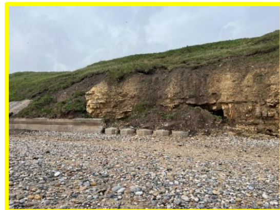
Minor outflanking to low level wall. Low beach levels exposing concrete blocks. (/0102C01)
