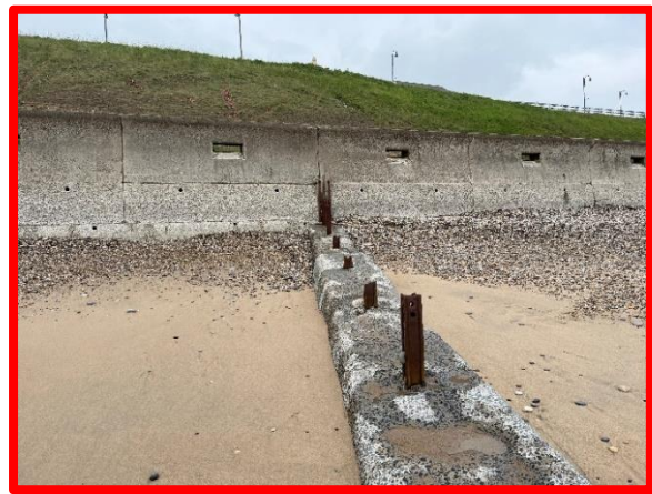
Remnants of derelict groynes (/0102C01)
