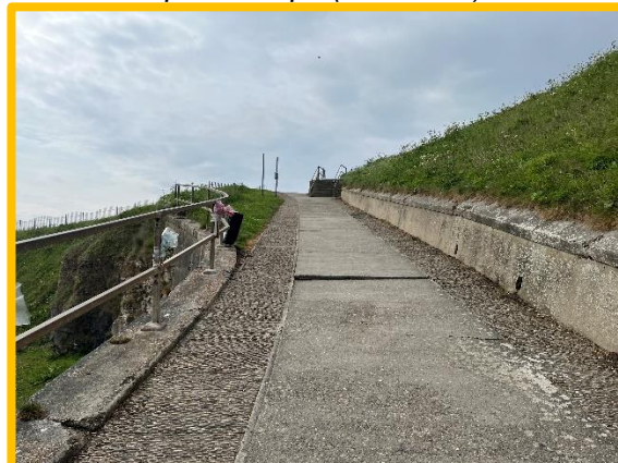
Movement of deck slabs in access ramp (/0103C07)
