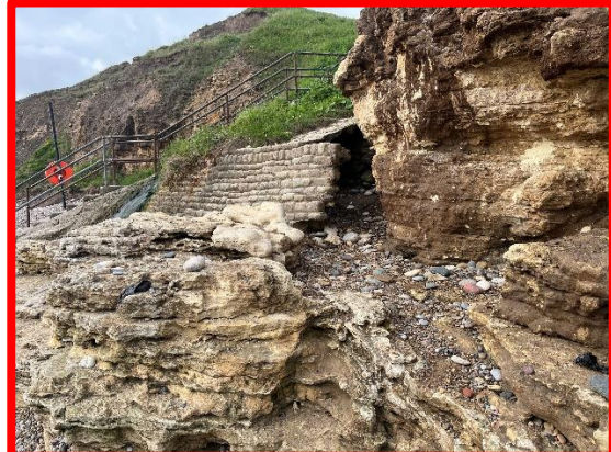
Outflanking of revetment causing washout of fill (/0804C01)
