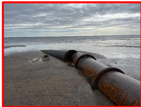
Failed large cast iron outfall (/0202C02)
