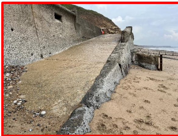
Hole in deck of ramp and exposed reinforcement (/0102C01)
