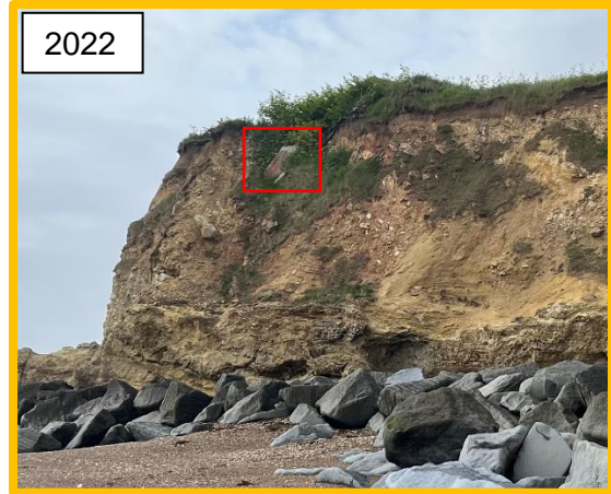
Erosion affecting fence line of properties to south Dawdon Dene Outfall - 2020 (/0103C02)
