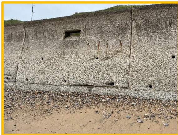
Spalling of bullnose on sea wall to the south (/0102C01)
