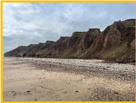
Glacial Till slumping along the majority of the frontage (/0804C01)
