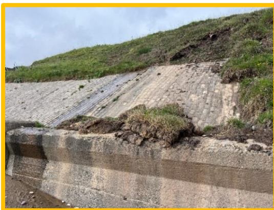
Bulging blockwork revetment and small slippage of till above. (/0102C01)
