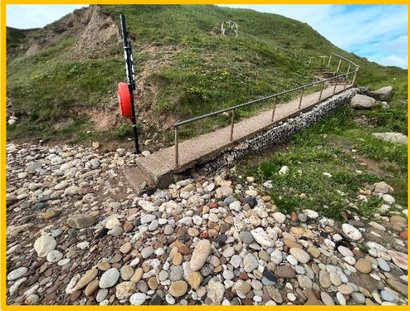
Gabion baskets retaining access ramp in poor condition (/0301C01)
