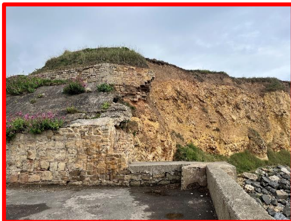
Masonry wall and concrete revetment at tie-in to cliffs breaking-up (/0103C04)
