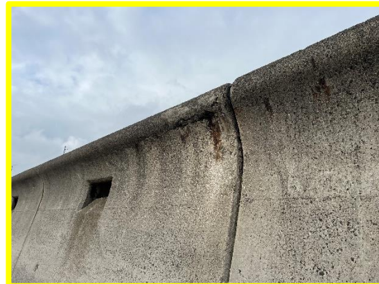
Horizontal cracking to bullnose (/0102C01)
