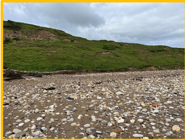
Former mouth of Castle Eden Dene eroding channel through foreshore and undercutting cliff toe. (/0202C02)
