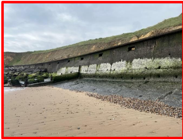
High beach levels concealing failed section of concrete apron identified in 2020 (/0102C01)
