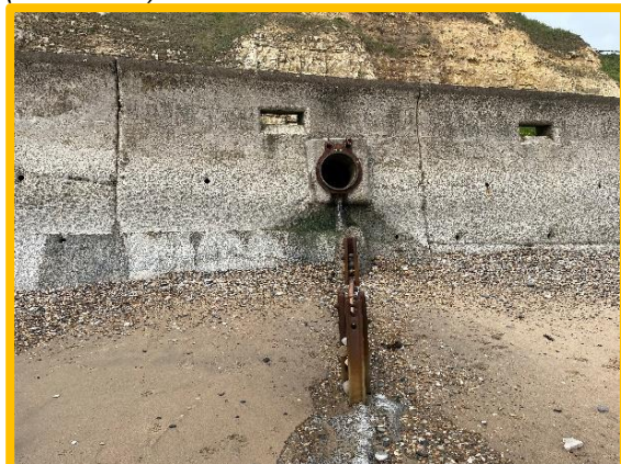
Missing cast iron flap valve (/0102C01)
